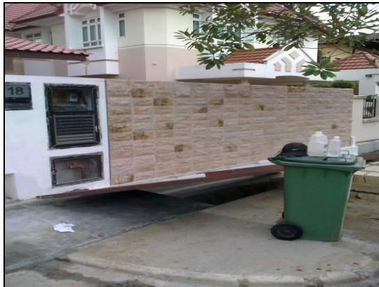
Photo showing the toppled incident gate
