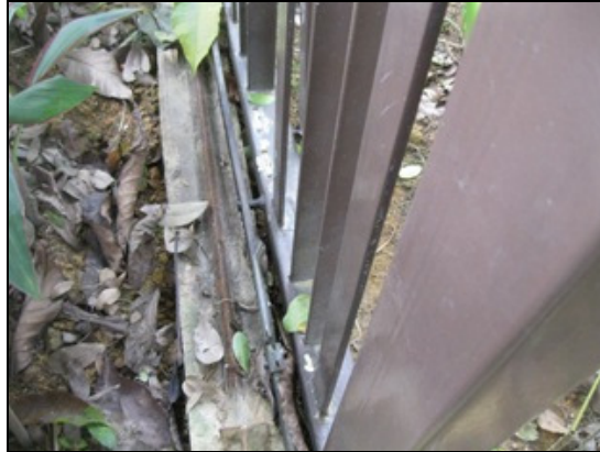
Photo showing the wheels of the incident gate not resting on the track
