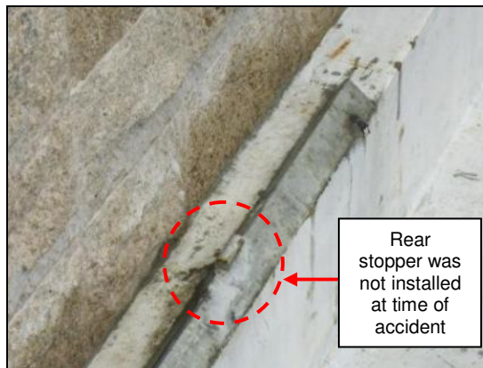
Photo showing the toppled incident gate
