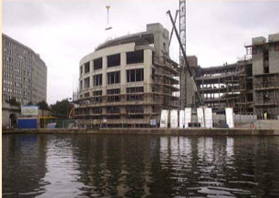
Precast cladding was selected for its buildability advantages, which were particularly important at this tight site.
