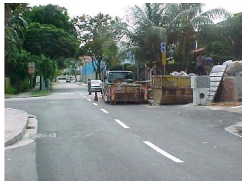
Skip on public street - endanger road users
