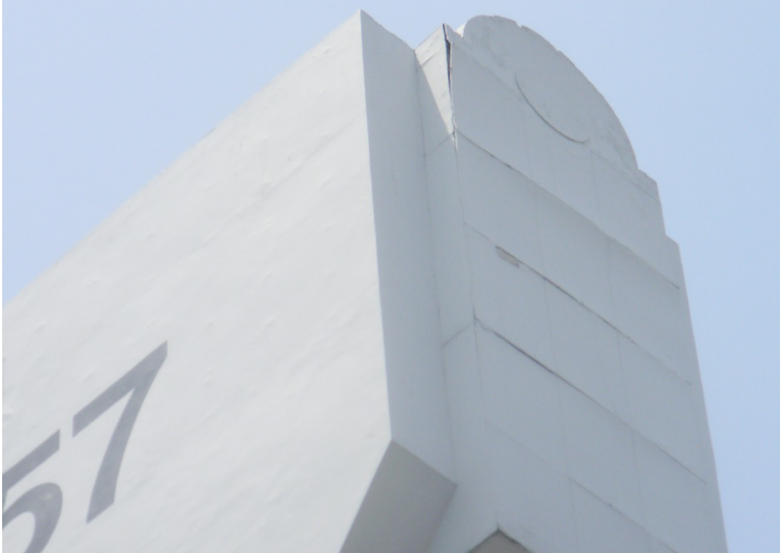
Example 1: Deteriorated calcium silicate board on exterior wall of building
