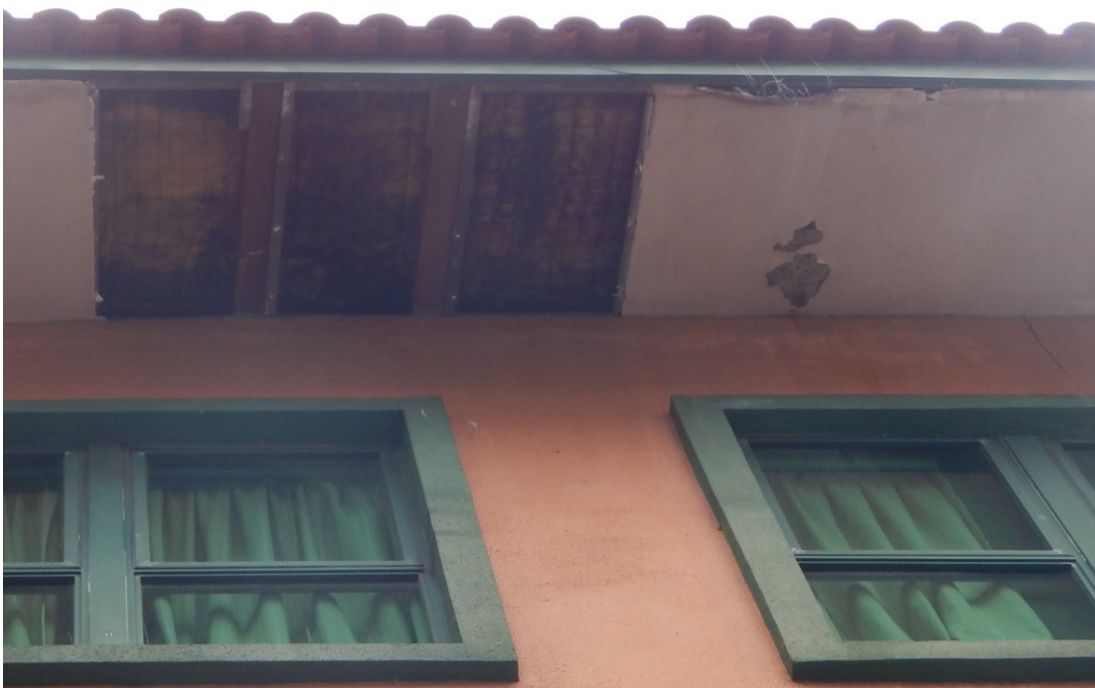
Example 2: Deteriorated gypsum board used as ceiling panels underneath of roof eave of building
