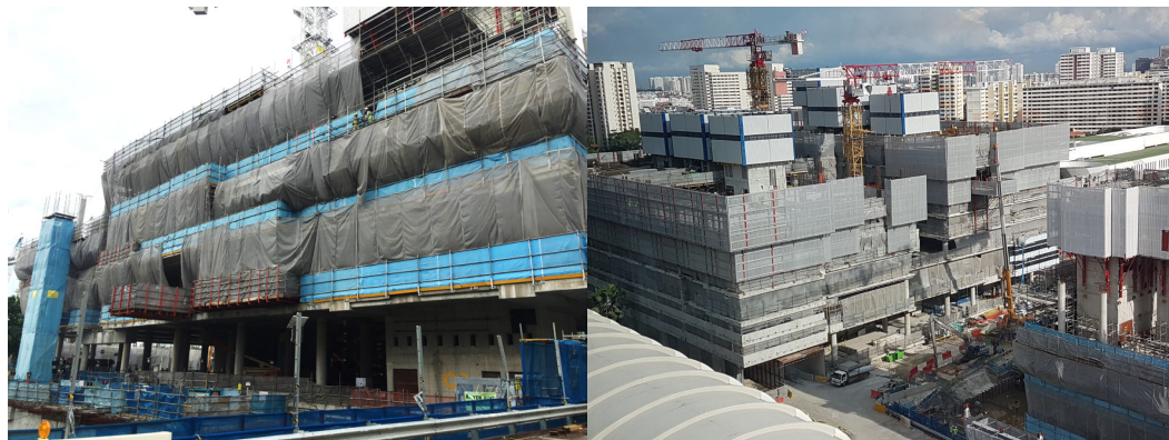
Site safety. Example of safety risks include falls from height. Being able to detect these hazards in a virtual model allows a project team to accurately plan necessary safety measures and locate placement of safety barriers as the project moves phase by phase.
