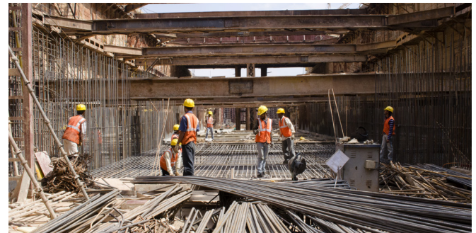
Interfacing between temporary and permanent works. Another critical point of consideration as the project progresses is sequenced interfacing between the temporary structures required or installed at that particular phase and the permanent works to be erected (e.g. a lift wall). A situation may arise on site where the permanent works are scheduled to be constructed but temporary works are still in place, thereby requiring more time, resource, and manpower in the workaround or rectification of the problem.
