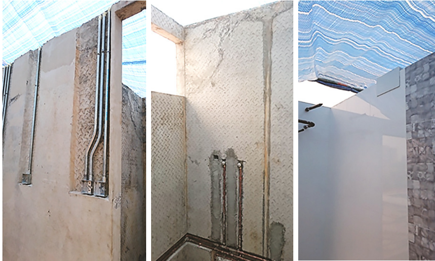
Over-provision of recess for electrical conduits
