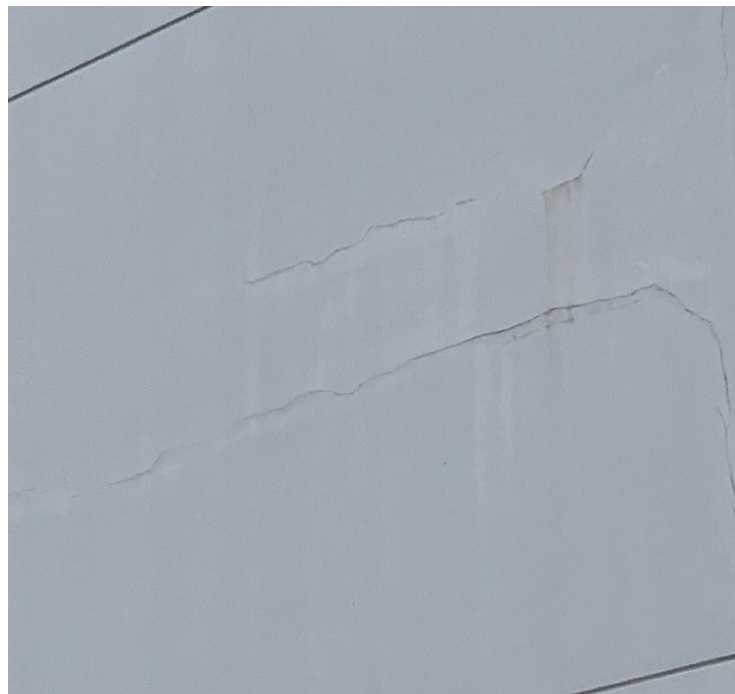
Figure 4: Interface cracks on external non-load bearing wall with no joint treatment
