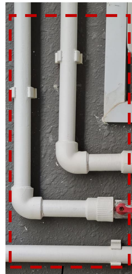
Close-up view of painted PPR water service pipes.
