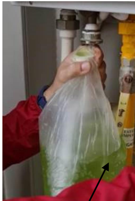
Algae in water from service pipe
