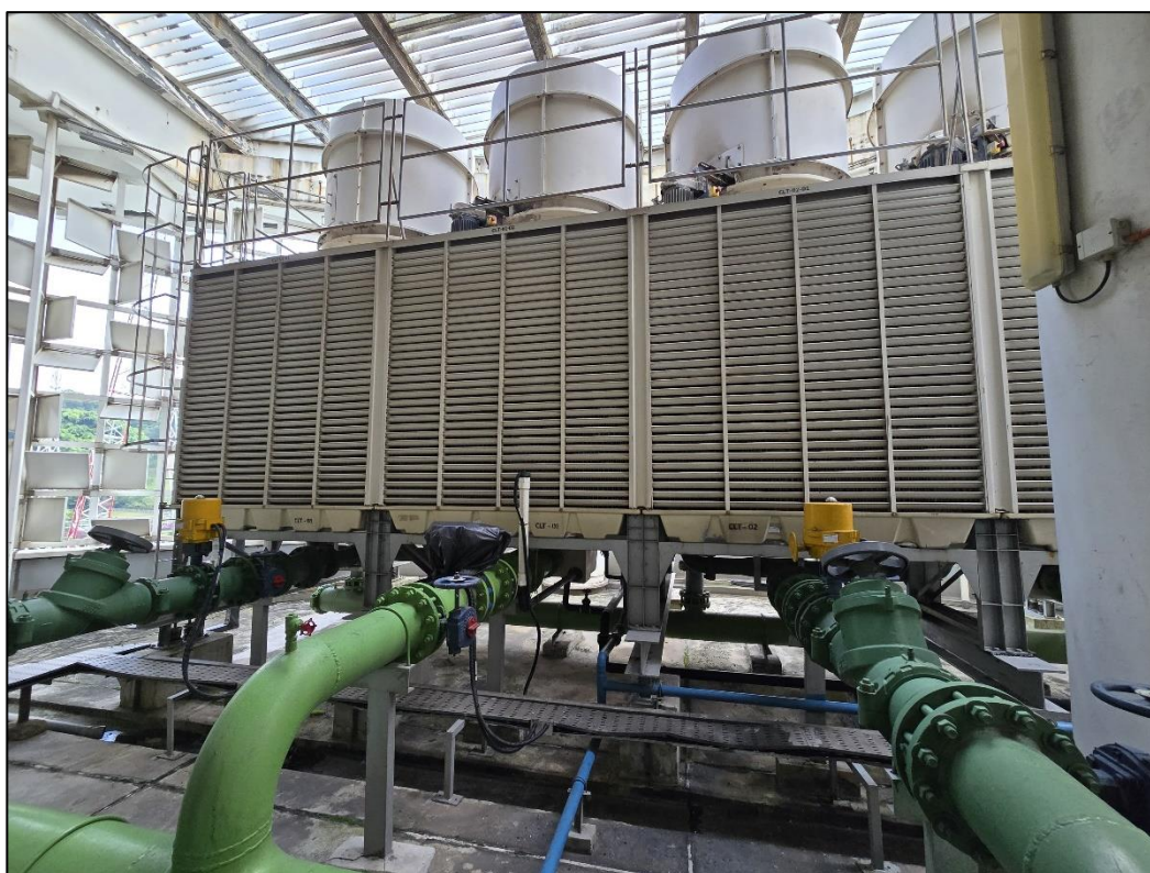
Example of tested and commissioned cooling tower
